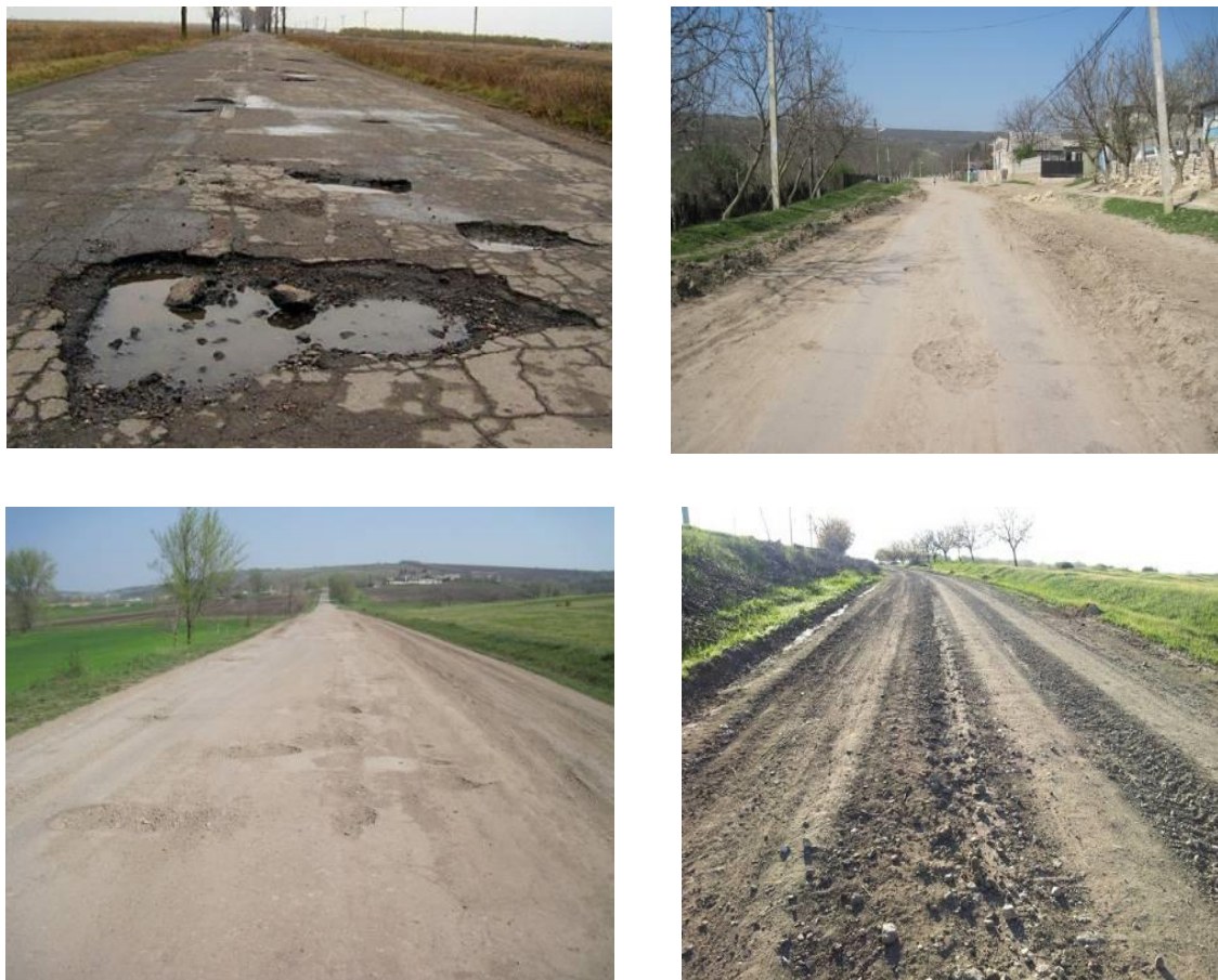
Figure 2-10: Damage to local roads
